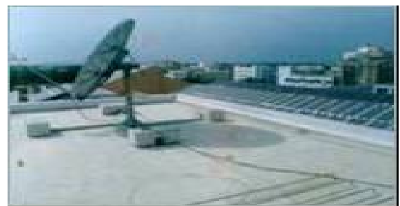
Roof top solar PV plant
